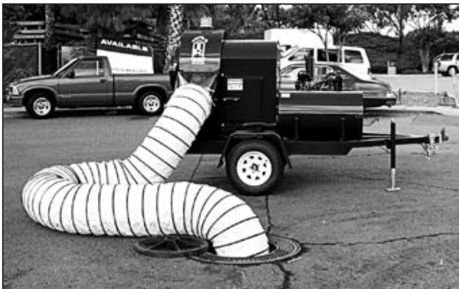
This ventilator, in Southern Calif., is powered by a large gasoline engine, and will generate almost 20,000 cubic feet per minute of airflow.
