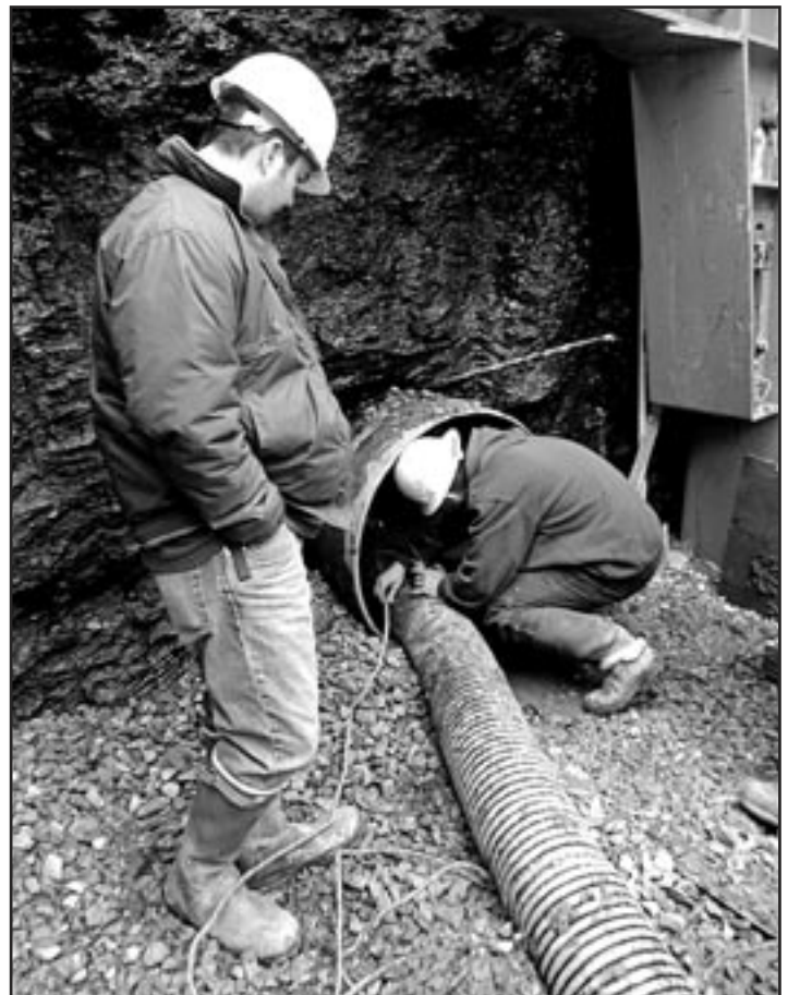
This contractor continuously ventilated this confined space during a water line inspection in North Little Rock, Ark., and the people who entered the space each carried an atmospheric gas monitor. A retrieval system, using anklets and lifelines, was also set up so that the workers could be pulled to safety in the event of an emergency.
